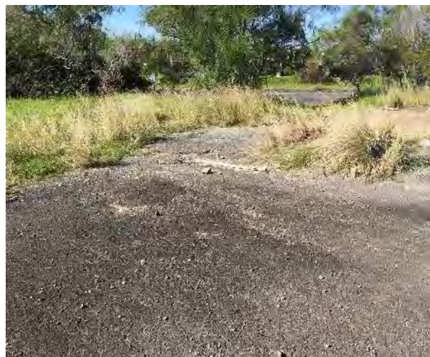
Figure 8 Bitumen and gravel surface across much of the site – former car park
