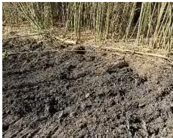
Figure 21 Removal of the bamboo and a maximum of 30cm of top soil
