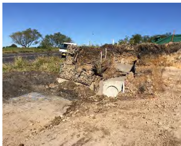
Figure 12 Removal of the gabion wall on the eastern boundary of the site for new access
