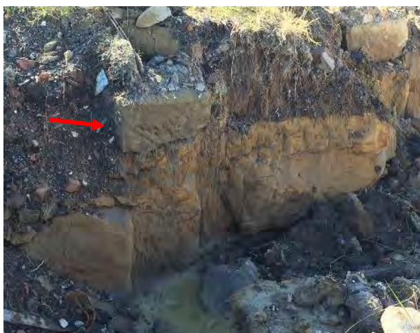
Figure 18 Section showing stone foundation of the Superintendent's house constructed onto natural clay bedrock
