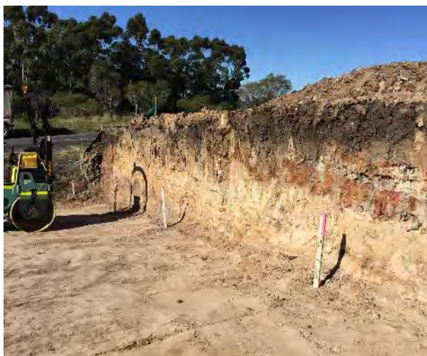
Figure 22 Excavation through topsoil and bedrock for the access driveway to Murray Dwyer Circuit on the eastern boundary
