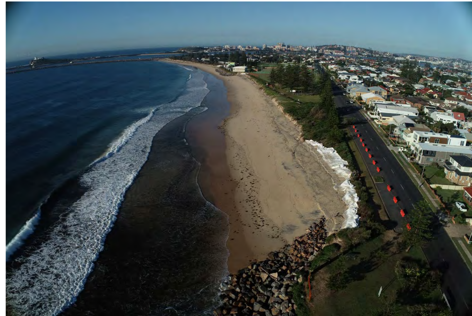
Picture 3: Emergency Sandbag Protection Works at the Southern End of the Mitchell Street Seawall. May 2020
