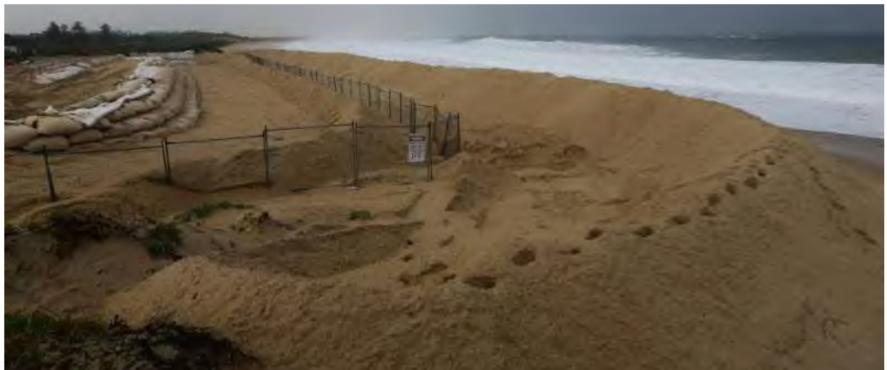
Figure 8: Construction of sea wall in front of the Hunter Water site (Source: Newcastle Herald, 2019).
