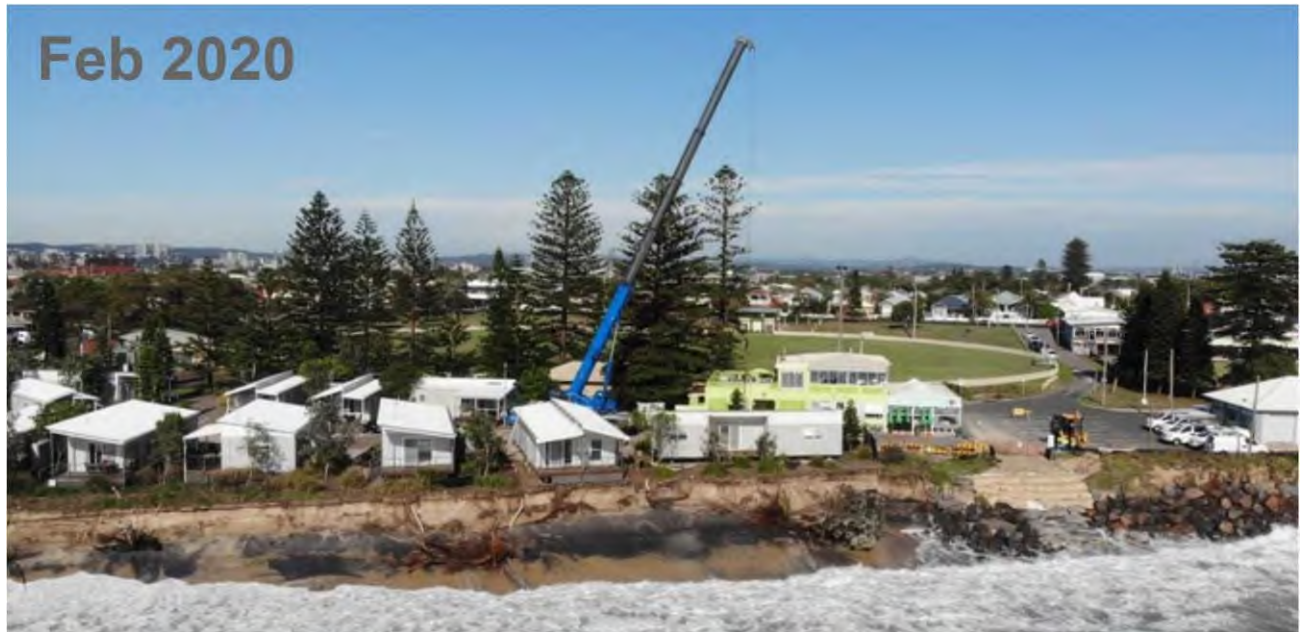
Figure 5: Cabins being removed from the caravan park due to beach erosion following a large wave event in February 2020 (source: M. Bardsley).
