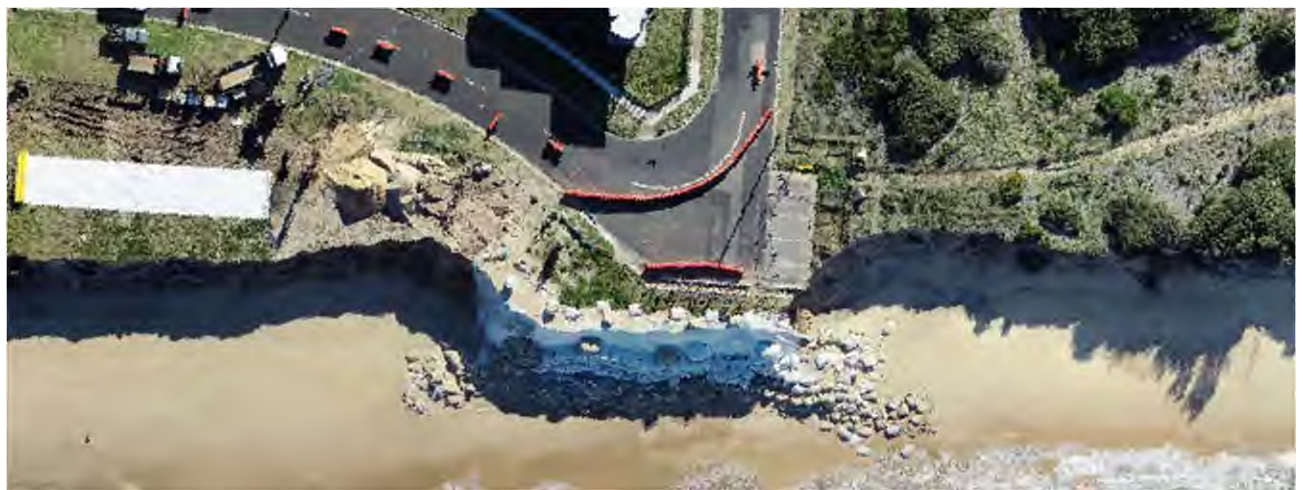
Figure 6: Erosion scarp and failing emergency coastal protection works at Griffith Ave (north of the Mitchell Street seawall) following an east coast low around the 15th July 2020 (source: CN).
