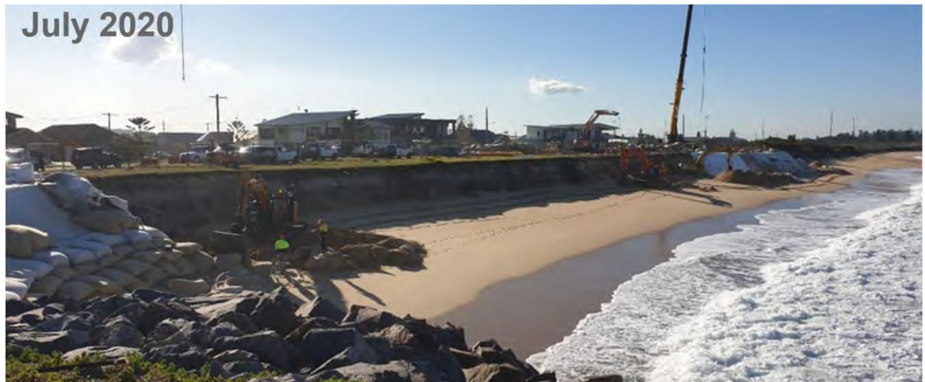
Figure 7: Emergency coastal protection works underway north of SSLSC seawall in preparation for a second east coast low in late July 2020 (source: M. Bardsley).
