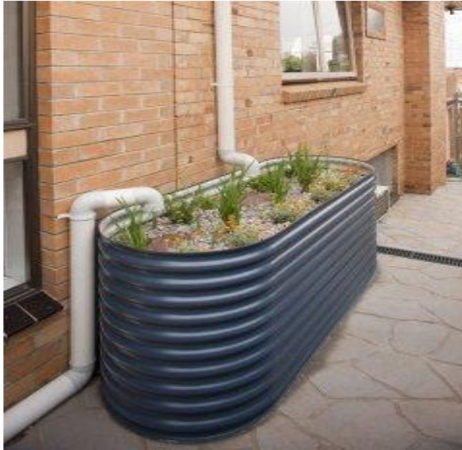
Figure 4.6.3 - Example of an above ground rain garden (Source: Water Services Association of Australia)
