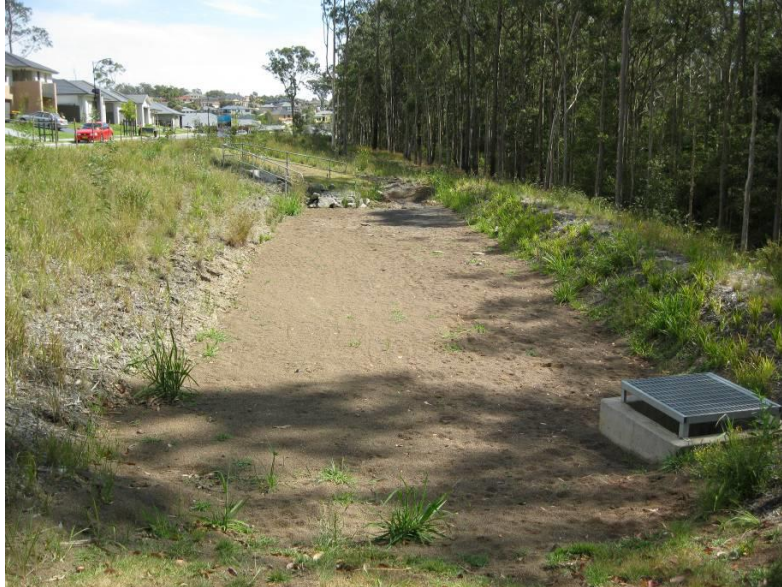
Figure 4.9.1 - Sand filter within basin
