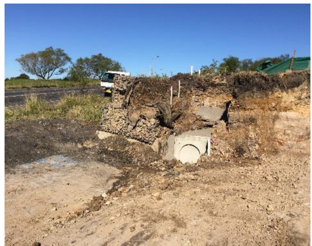
Figure 12 Removal of the gabion wall on the eastern boundary of the site for new access
