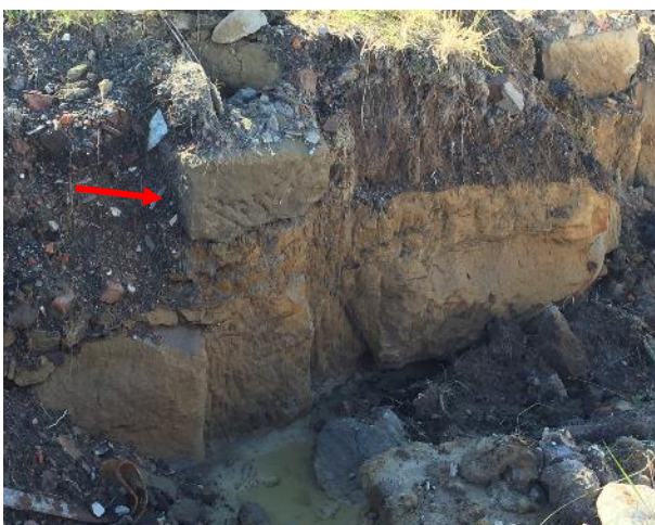
Figure 18 Section showing stone foundation of the Superintendent's house constructed onto natural clay bedrock
