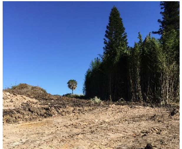
Figure 23 View west at the top of the access driveway and remnant stand of bamboo
