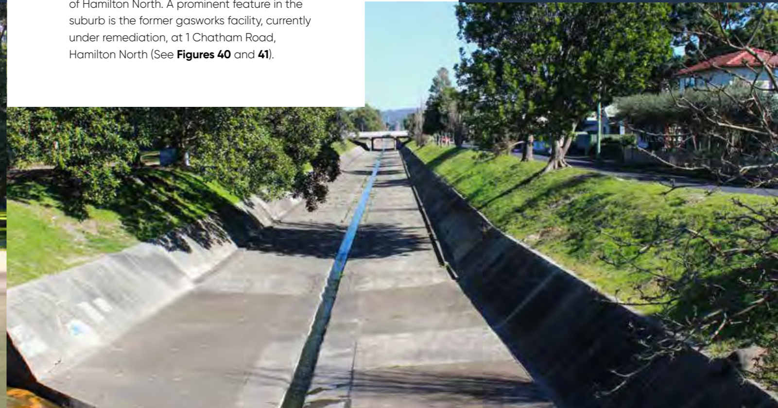
Figure 40. Styx Creek (stormwater channel) looking west to Broadmeadow from Chatham Road, Hamilton North. (Photograph: MManning, CN, 21/7/19).
