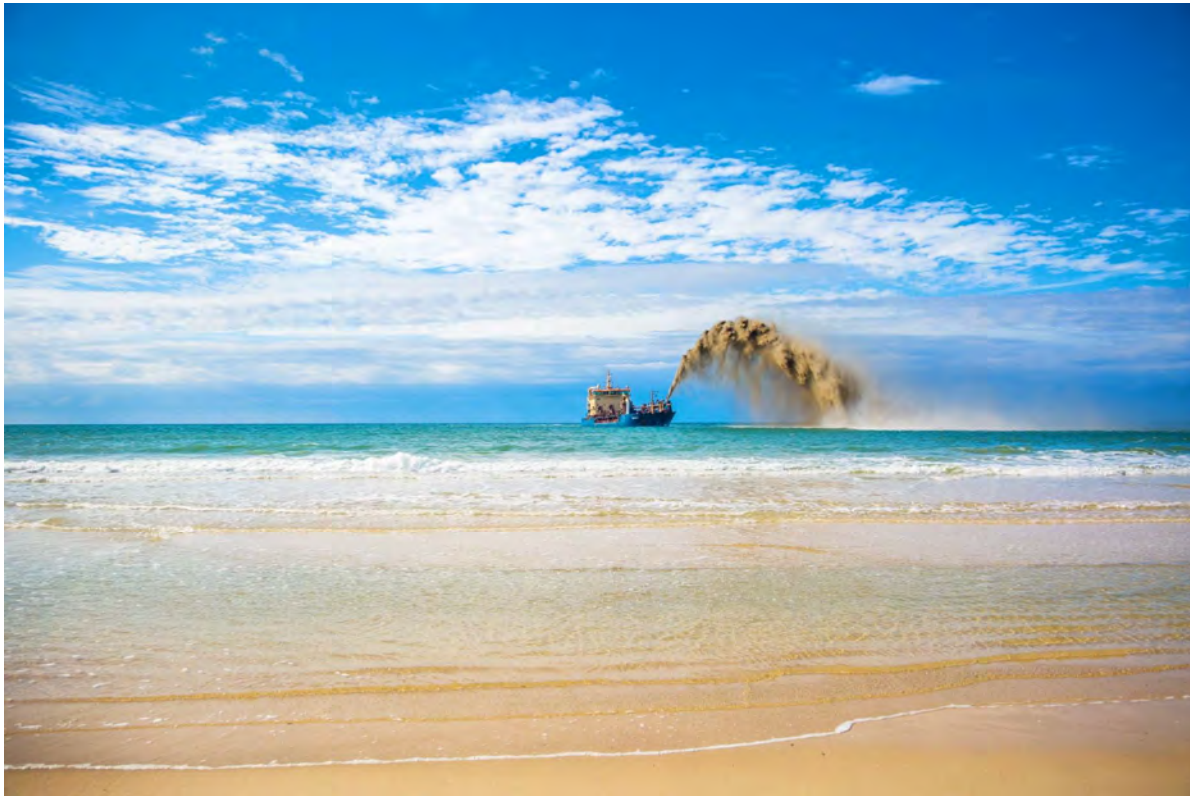
Figure 4: A TSHD rainbowing sand onto the nearshore area of the beach as part of beach nourishment works (source: City of Gold Coast).
