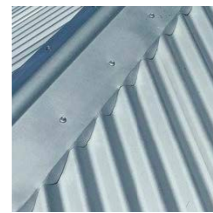
Unpainted corrugated metal roof sheeting, flashing and downpipes to all new and replaced roofs
