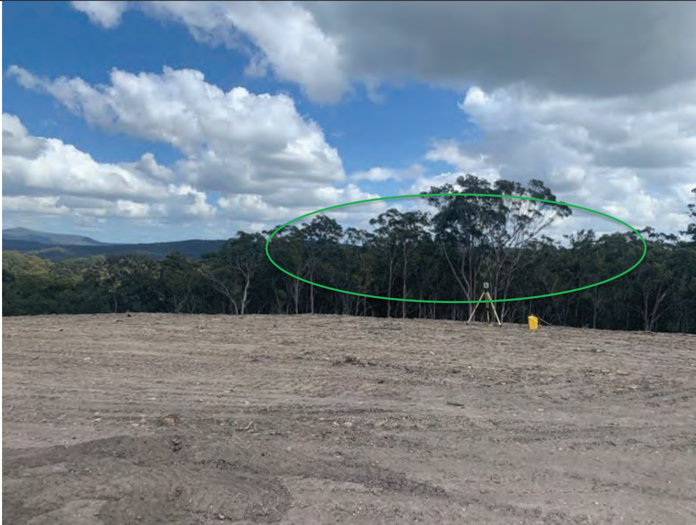
Photo taken from future Walker Crescent, Fletcher looking directly north over the site
