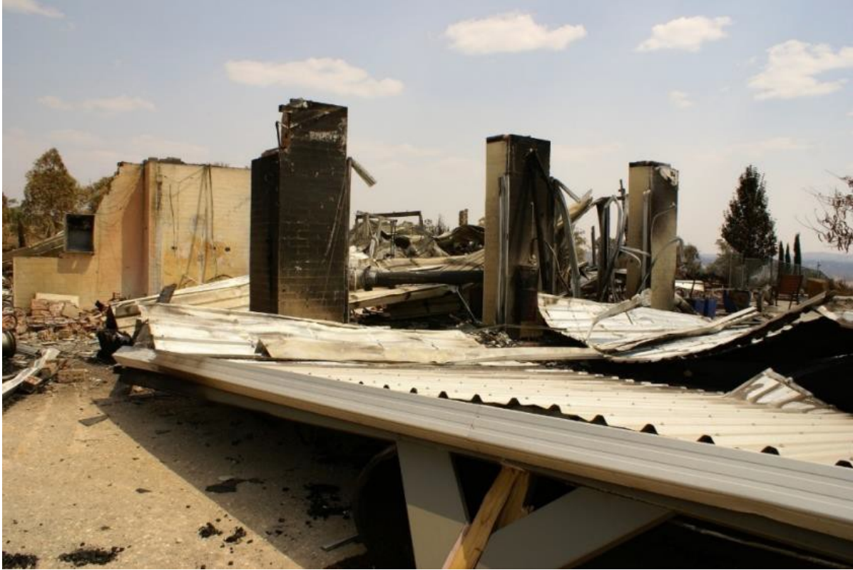
Infrastructure damage during the 2019-2020 Australian bushfire season. Picture by Mark J Toomey, Pixabay.
