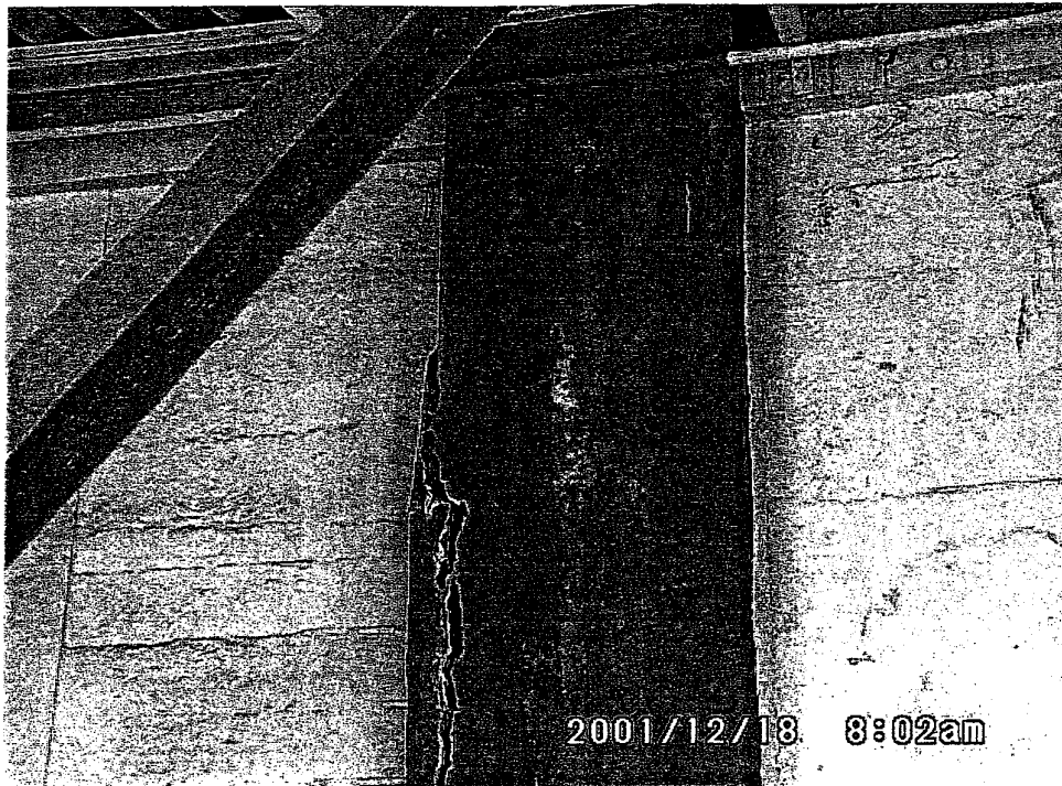
Photograph 12180017 Cracking in column on reverse, associated with low cover
