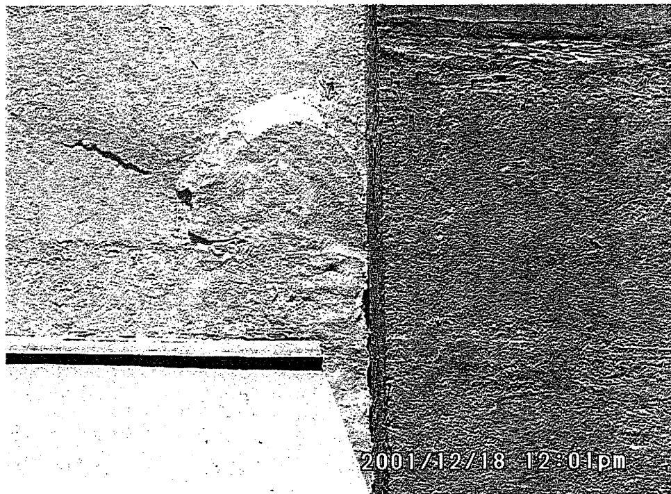
Photograph 12180102 Close-up of bulge in front facade indicating imminent spall
