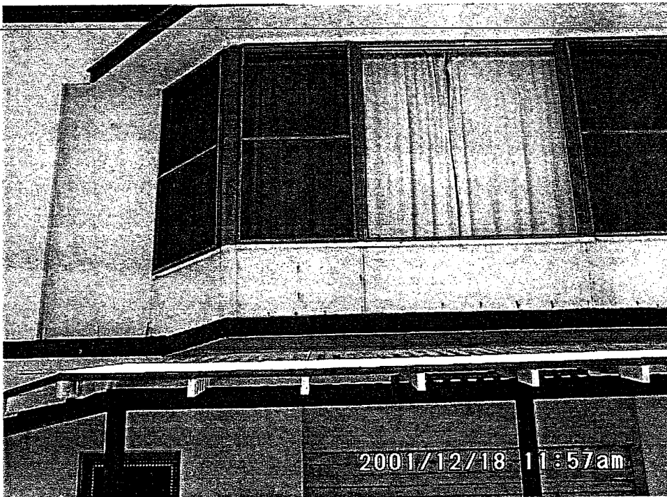
Photograph 12180086 Corroding fixtures in rear façade of residence
