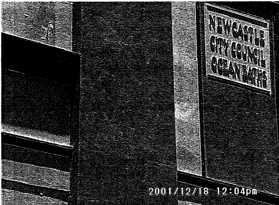
Photograph 12180112 Bulges in front facade indicating imminent spalls
