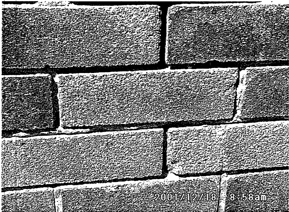
Photograph 12180034 Salt fretting of some bricks
