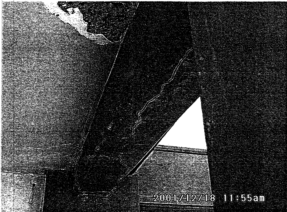
Photograph 12180079 Cracking in beam to colonnade
