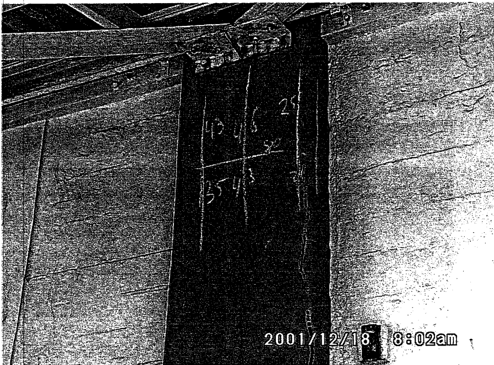
Photograph 12180016 Cracking in column on reverse, associated with low cover
