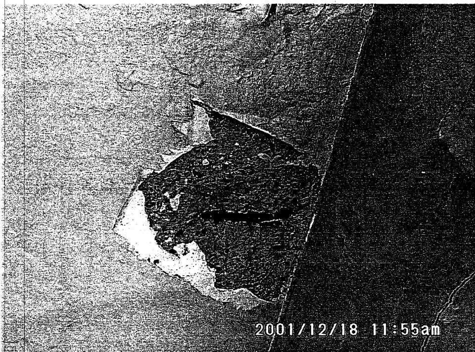
Photograph 12180080 Spalling in roof slab soffit to colonnade
