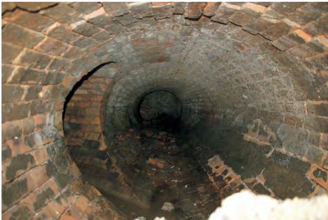
The Church Street Drain, possibly looking west along Church Street, with a branch of the drain going under the Courthouse (Bill Jordan, 2008).
