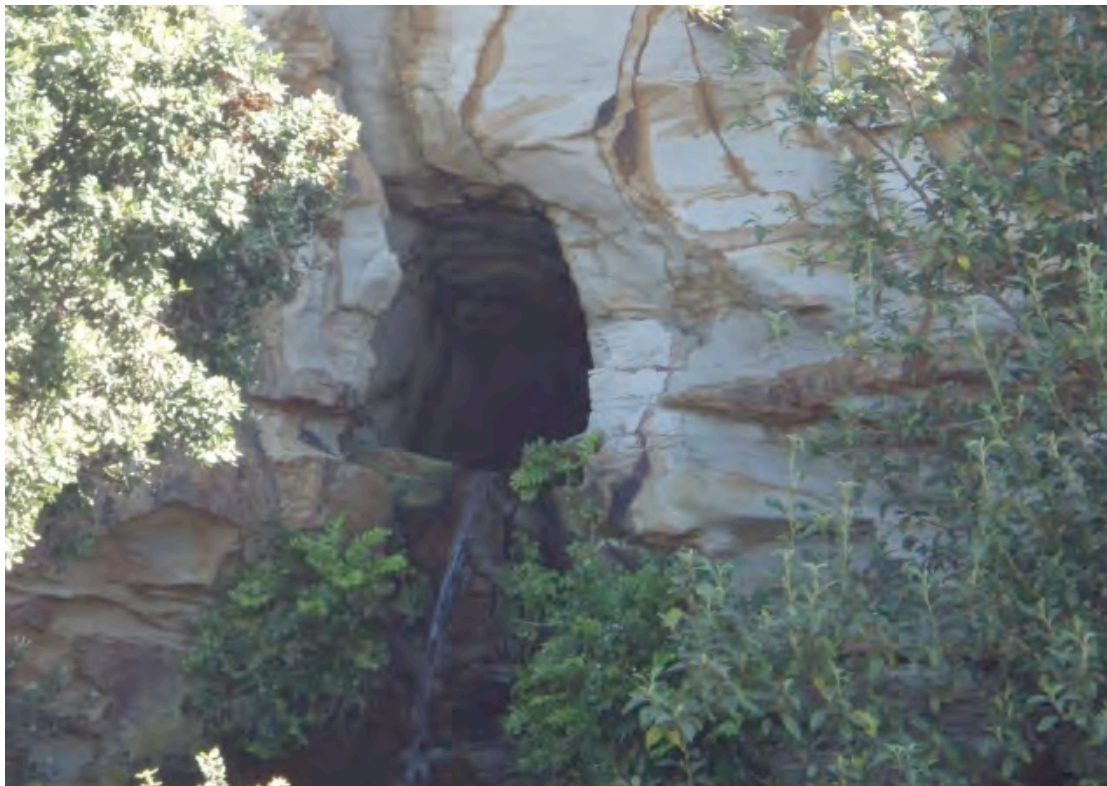
Outfall of the Church Street Drain above Shortland Esplanade (Newcastle City Council Road Asset (RA) 17).
