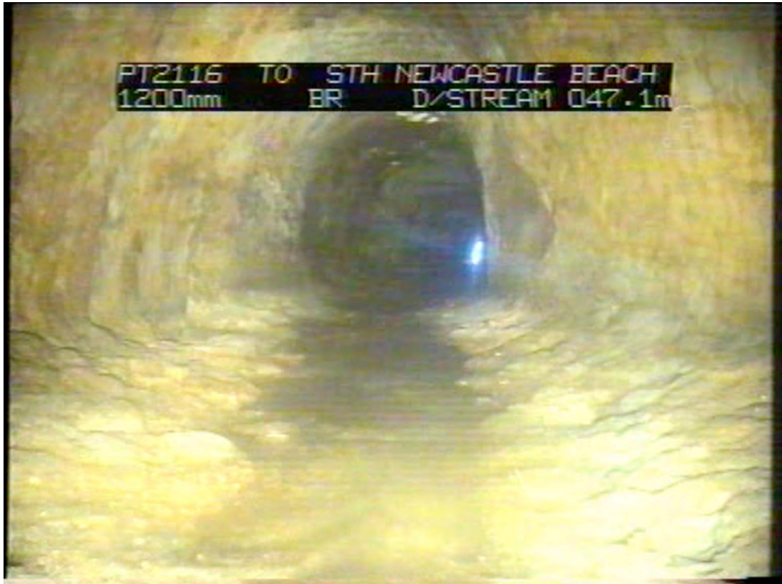
Section of the stone adit under Church Street, looking east to outfall (Newcastle City Council Road Asset (RA) 17).
