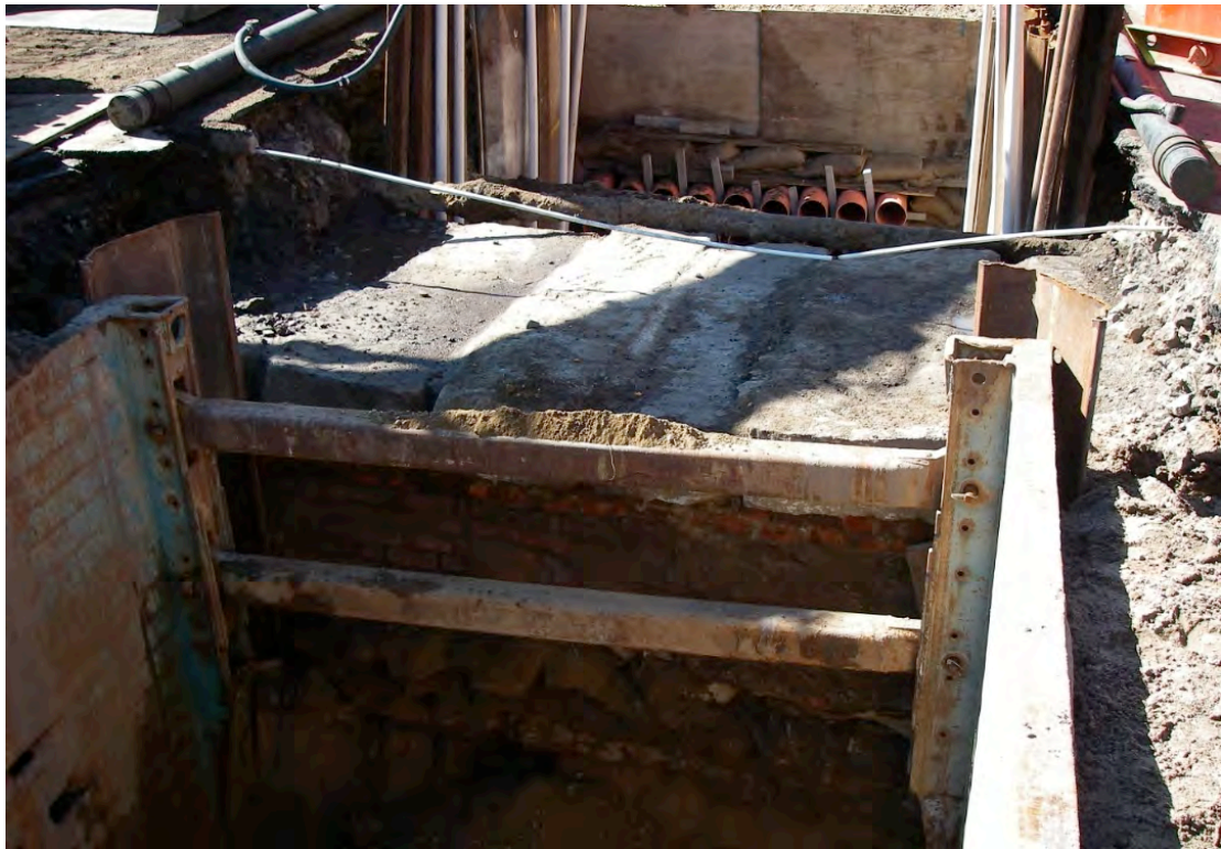
The Darby Street Drain in the vicinity of Tyrrell Street. Note the sandstone slabs forming the lid of the drain (Newcastle City Council Road Asset (RA) 20).
