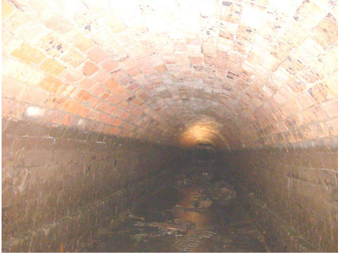
Brick arch drain, on the north side of the railway near Centenary Road and Argyle Street (Newcastle City Council).
