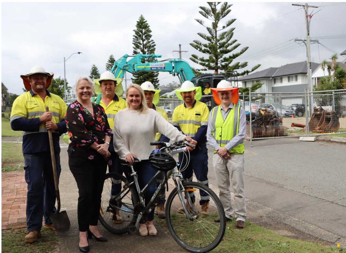
Councillor Carol Duncan and Newcastle Lord Mayor Nuatali Nelmes celebrate the start of the cycleway's construction with workers at the site
