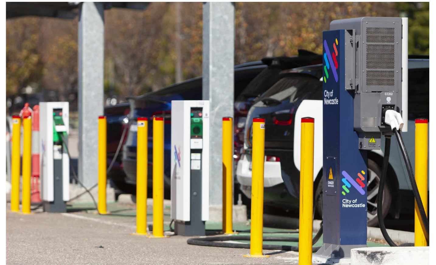
Electric Vehicle (EV) charging station, No.2 Sportsground.
