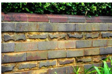
Textured face brick fencing. Fencing in face brick with curved edges and geometric patterns was popular in the Garden Suburb during the Inter-War era.
